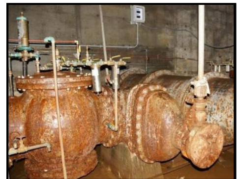
Tunnel valves in need of repair
